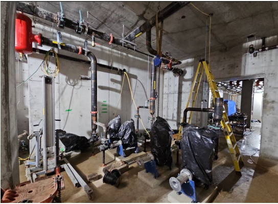
Pump hook-up in new mech room – February 2024
