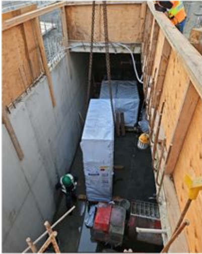
Delivery of mechanical equipment - November 2023
